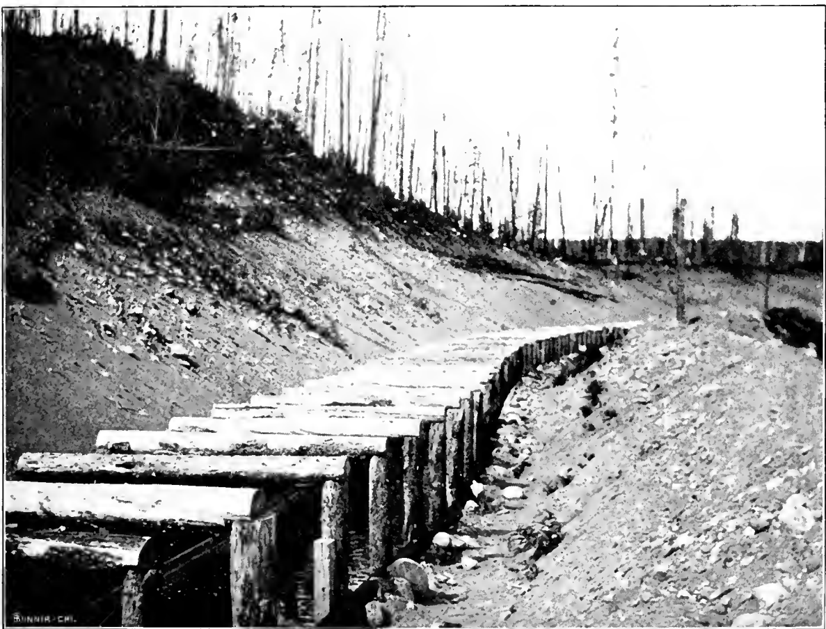
SHOWING DITCH THROUGH BAD GROUND. 43RD COMPANY'S FLUME AND DITCHES—OMINECA M. D.
